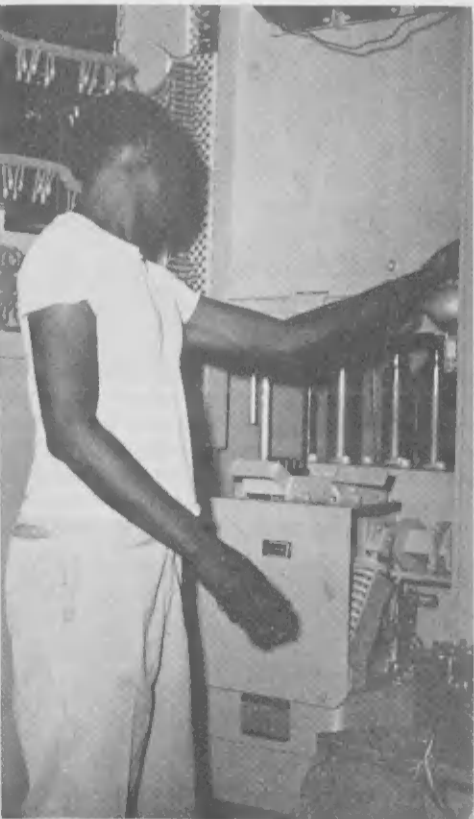
WHEN THE facilities of the substation had been checked out, the air circuit breaker on a Lago feeder was moved from its testing to operating position. ORA CU e facilidadnan di e substacion a worde gecheck, e interruptor di aire ariba un cable di Lago a worde moví for di su posicion di test pa posicion di operacion.
